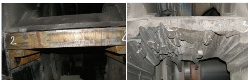
Fig. 1. Condition of the coal grinding plates within the mill immediately after replacement, when they are new (left) and immediately before replacement, when they are depleted (right)
