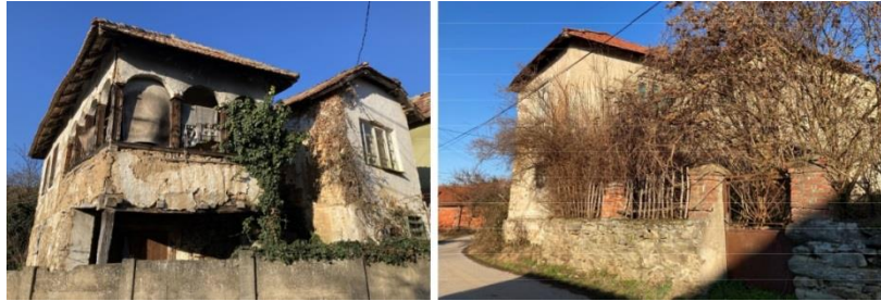
Fig. 7 Old and abandoned village houses and their facades Source: author's recordings (March 2021)
