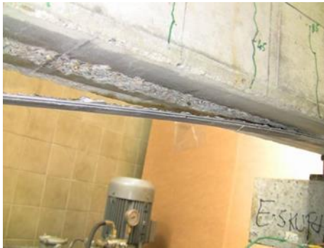
Fig. 6 Loss of bond between concrete and epoxy adhesive
