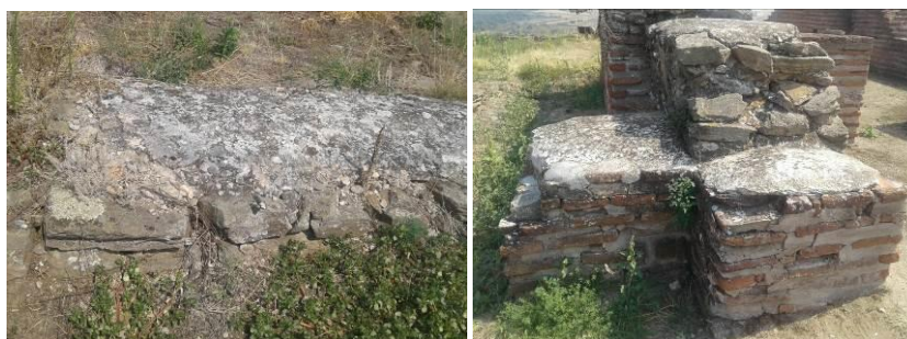
Fig. 12 Inadequate concrete “caps” (photo: A. M. Petronijević)
