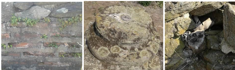
Fig. 11 Vegetation in the damaged bricks (left); lichen on the parts of a stone plastics (middle); cut tree at the base of the wall (right) (photo: A. M. Petronijević)
