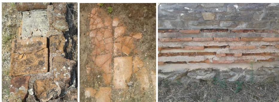
Fig. 7 A detail of brick pavement – the brick is cracked (left); poor quality bricks used for conservation (photo: A.M.Petronijević)
