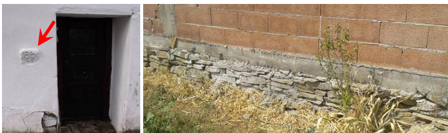
Fig. 13 a) Pieces of stone plastics from Caričin Grad built into St. Ilija church (photo: Institute for Cultural Heritage Preservation of Niš), stone from the site built into the foundations of the walls of surrounding buildings (photo: A.M.Petronijević)
