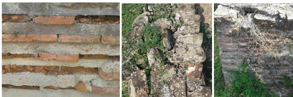
Fig. 10 Degradation of bricks, and mortar after conservation (photo. A.M.Petronijević)
