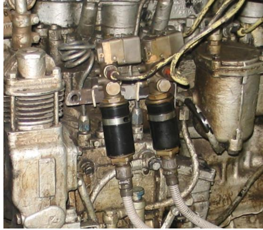
Fig. 2 Fuel system of the D-240 engine with solenoid valves to turn off the fuel supply of two ICE cylinders
