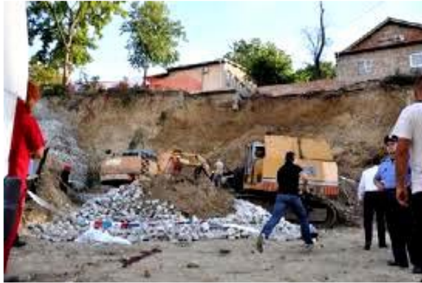
Fig. 6 Retaining wall collapse at a construction site in Zemun, Serbia [2]
