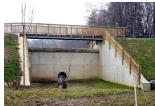
B. Retention basin Am Eichengrund.
