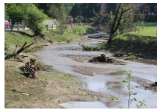
B. Widening the stream bed in the area of the Gasthof Pflieger. http://www.freiland.at/de/hws_schoeckelbach/
