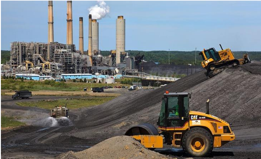
Fig. 3 Storage and maintenance of fly ash in a power plant
