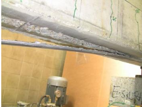
Fig. 6 Loss of bond between concrete and epoxy adhesive
