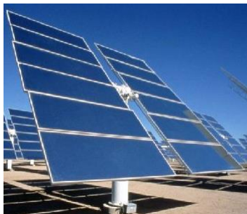
Fig. 3 An example of a ground mounted system
