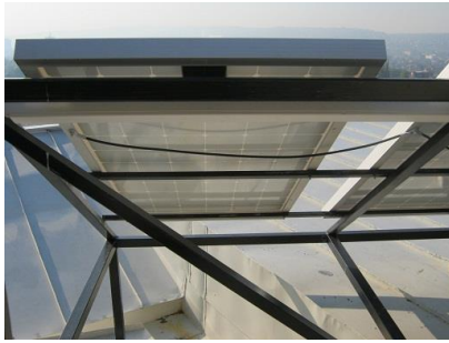
Fig. 7 Fixed photovoltaic system
