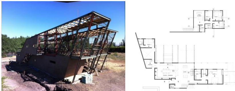
Fig. 2 The appearance of the house during construction, Santiago, Chile, the base of the ground floor and first floor, source 6
