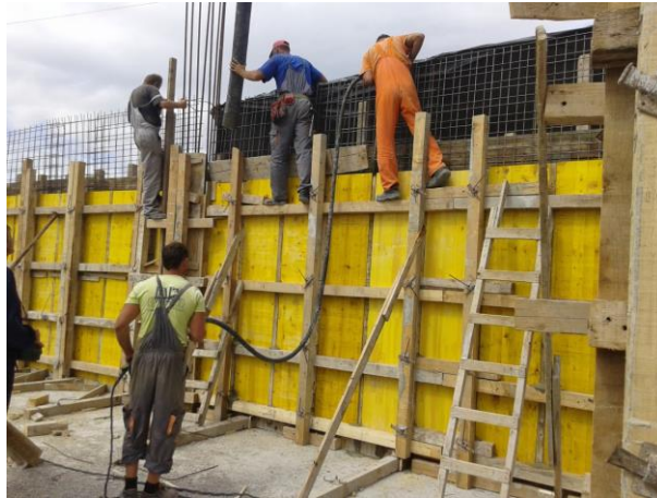
Fig. 3 Concreting of reinforced concrete walls (photo by the author of the paper)
