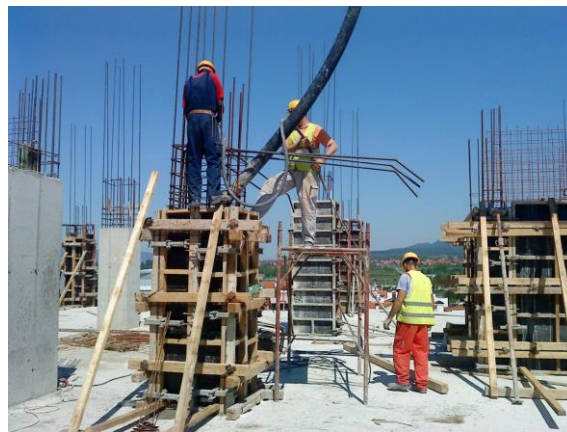
Fig. 2 Concreting of reinforced concrete columns (photo by the author of the paper)
