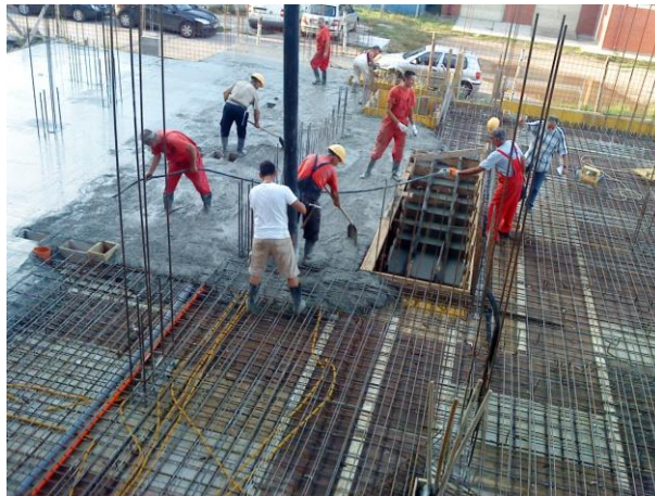
Fig. 4 Concreting of reinforced concrete slab (photo by the author of the paper)
