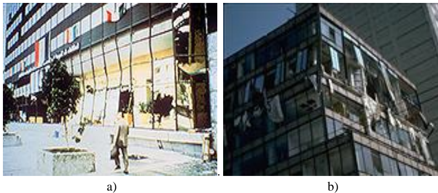
Fig. 2 Damages caused by Mexico earthquake, 1985
