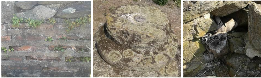
Fig. 11 Vegetation in the damaged bricks (left); lichen on the parts of a stone plastics (middle); cut tree at the base of the wall (right) (photo: A. M. Petronijević)
