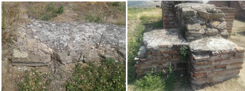
Fig. 12 Inadequate concrete “caps” (photo: A. M. Petronijević)
