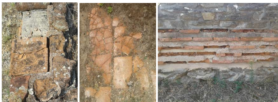
Fig. 7 A detail of brick pavement – the brick is cracked (left); poor quality bricks used for conservation (photo: A.M.Petronijević)
