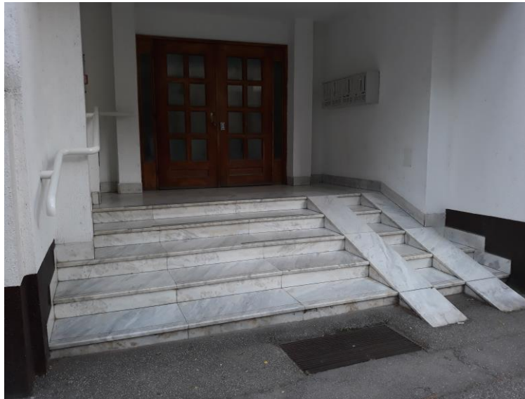
Fig. 3 Ramp which does not meet the standards (Photo: Branka Protić – Gava)
