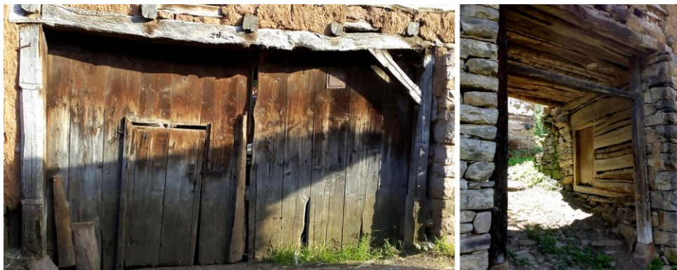
Fig. 4 Pedestrian entrance obtained by cutting in the great gate wing (photo I. Đorđević)
