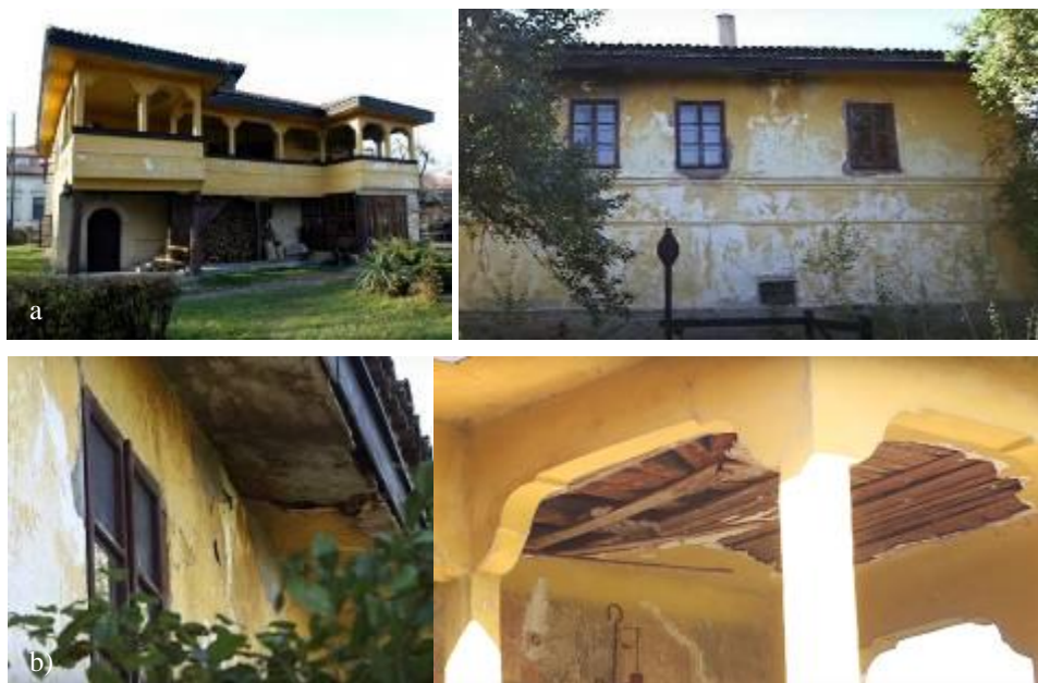
Fig. 3 Katić's house in Trstenik: a) Current condition of the exterior b) Katić's house in Trstenik: Visibly derelict façade and ceiling damage (Source: http://spomenicikulture.mi.sanu.ac.rs/spomenik.php?id=801 )
