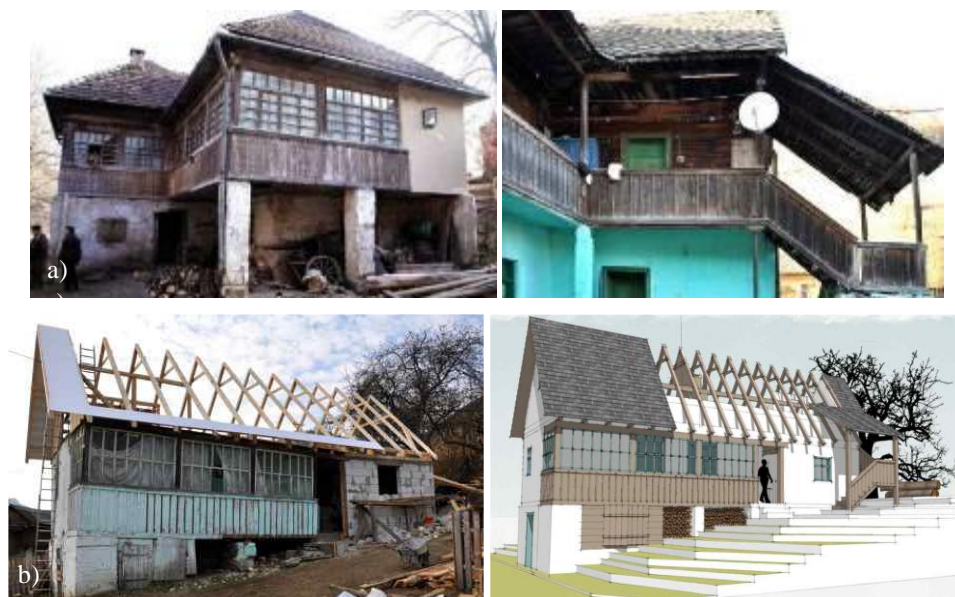
Fig. 7 Traditional houses in Tara Mator area: a) some of numerous houses which are still used, but inadequately treated; b) one of the examples of derelict houses, with the initiated renovation process, and the presentation of the possible solution (Barbieri, 2012)
