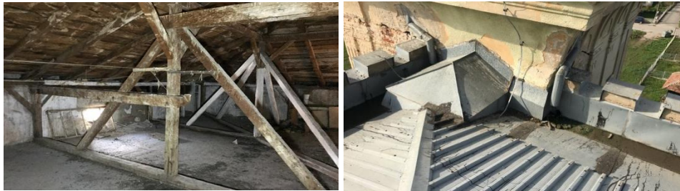
Fig. 5 “Karađorđev dom”, interior of the attic (left), damage caused by inappropriate roof reconstruction (right) author: E.V.Petrović (November 2020)
