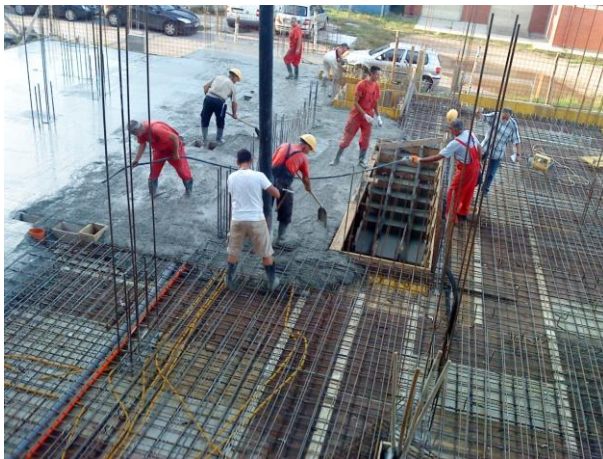
Fig. 4 Concreting of reinforced concrete slab (photo by the author of the paper)
