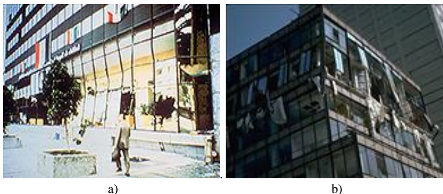
Fig. 2 Damages caused by Mexico earthquake, 1985
