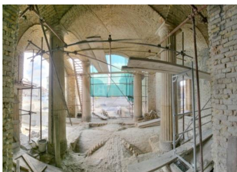
Fig. 4 Photograph of the vaults on the ground floor of hotel facilities in the “Pest Városhoz” building (photograph author: Photonino, www.subotica.info)
