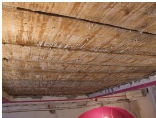
Fig. 5 Photograph of the ceiling made of timber half-cylinders on the ground floor of the former hotel “Hungaria” (photograph author: Viktorija Aladžić)
