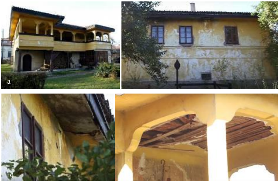
Fig. 3 Katić's house in Trstenik: a) Current condition of the exterior b) Katić's house in Trstenik: Visibly derelict façade and ceiling damage (Source: http://spomenicikulture.mi.sanu.ac.rs/spomenik.php?id=801 )
