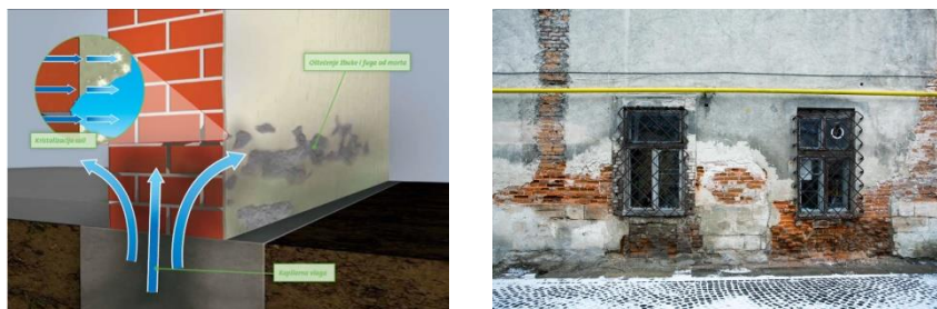
Fig. 4 Capillary moisture, initiator and cause of damage occurring on the walls and foundations [7]
