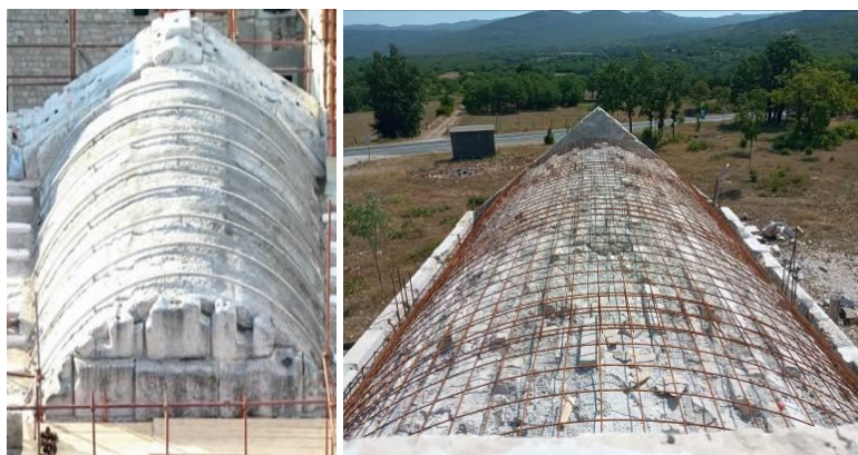
Fig. 15 a) Reinforcement of the vault extrados with steel arches, b) masonry vault reinforcement with additional RC vault (photo: P.P.)
