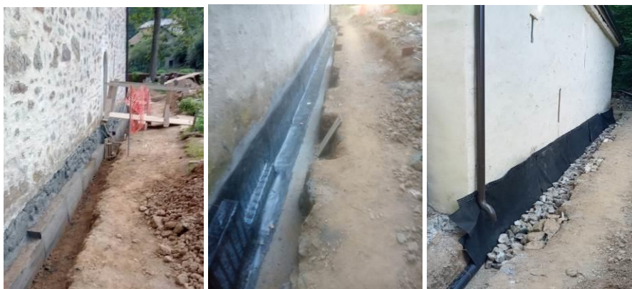
Fig. 13 a) reconstruction of the plinth wall, b) hydro-isolation, c) drainage (Photo P.P.)
