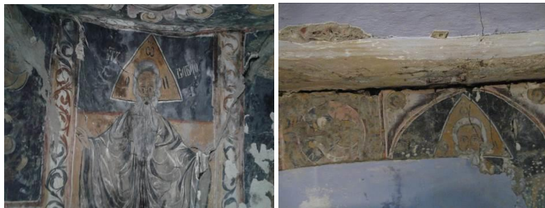
Fig. 4 Cracking in the barrel vault of the st. Nicholas church, (photo: P. Petronijević)
