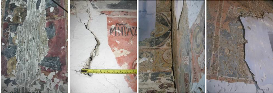
Fig. 9 characteristic cracks between the vault and the transverse walls (photo. P.P.)
