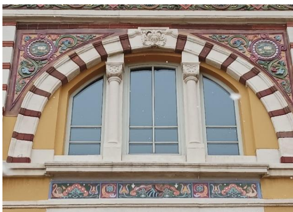
Fig. 12 Decorative panels with floral ornaments and water lily, central in the triangular panels near the triforia. Bottom a frieze with swans and beasts, Central Mineral baths, Sofia. Photography: Blagovesta Ivanova.
