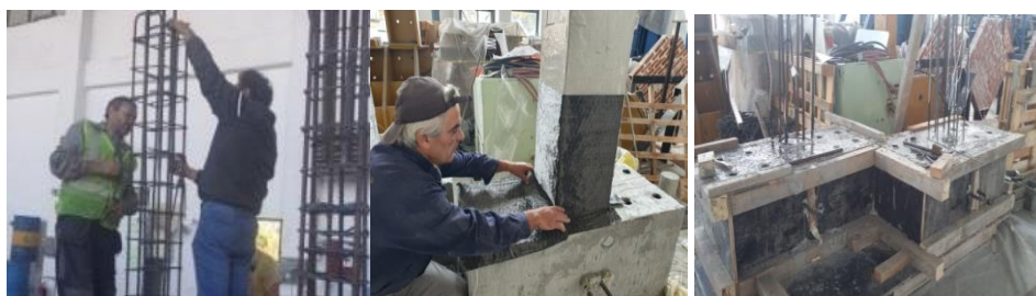
Fig. 1 Construction of the column models for experimental tests and Photos taken during application of FRP on the mode
