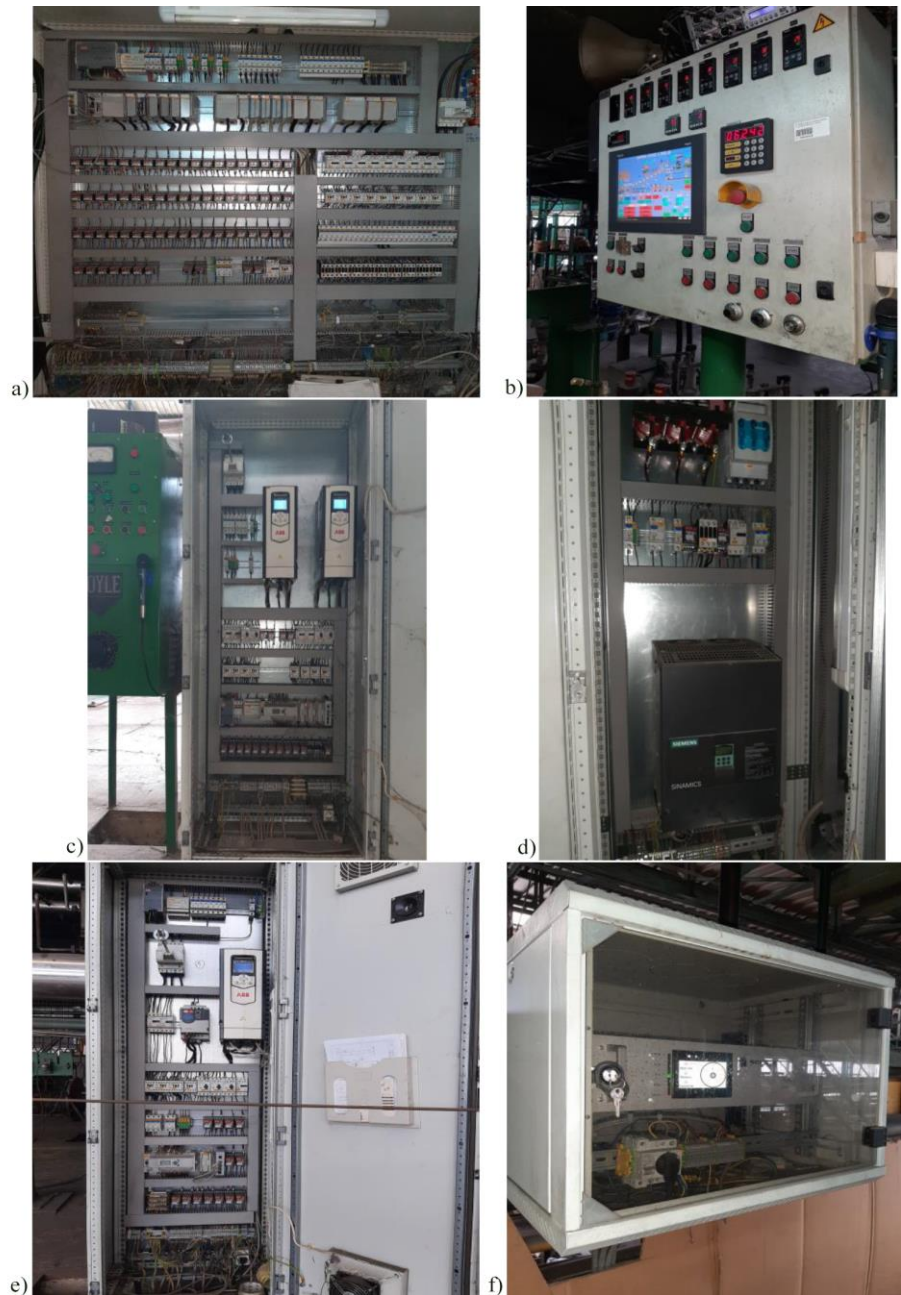
Fig. 5 a) Main control cabinet with CopmactLogix L35E PLC, b) main control desk with HMI panel, c) unwinder cabinet with ABB controllers and MicroLogix 1400 PLC, d) main traction device cabinet with Sinamics DCM converter, e) winder cabinet, f) cable position device cabinet Solz
