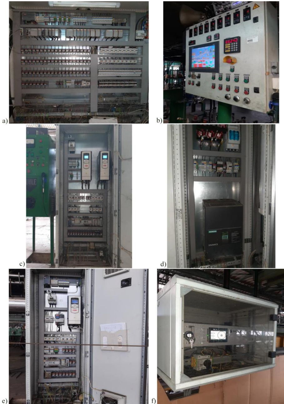
Fig. 5 a) Main control cabinet with CopmacLogix L35E PLC, b) main control desk with HMI panel, c) unwinder cabinet with ABB controllers and MicroLogix 1400 PLC, d) main traction device cabinet with Sinamics DCM converter, e) winder cabinet, f) cable position device cabinet Solz
