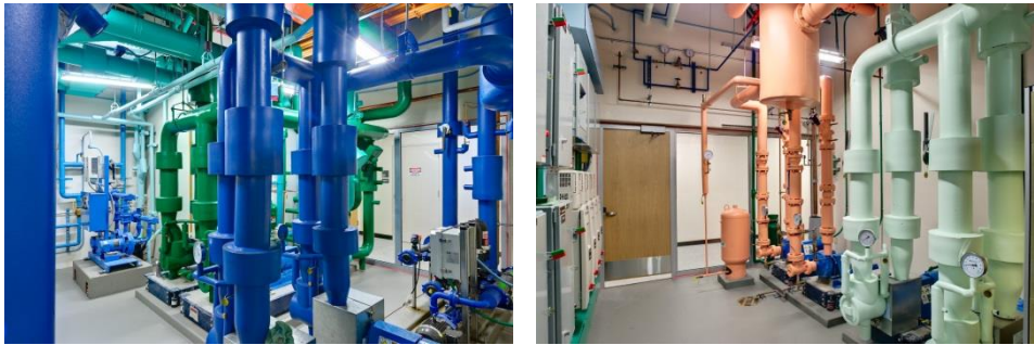
Fig. 2 Mechanical equipment, pumps, piping, and sensors
