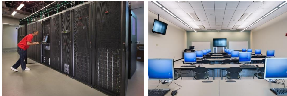
Fig. 6 (a) The Server room consist of private Cloud Computing System. (b) Computer laboratory connected to cloud computer using thin clients.
