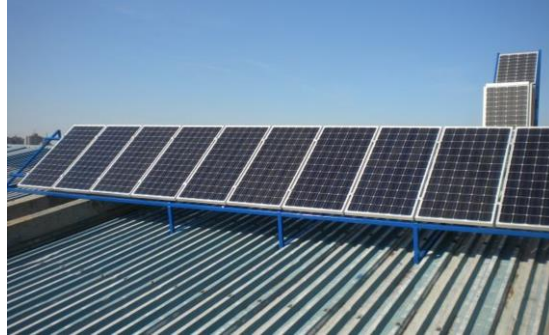
Fig. 2 A 2 kWp PV solar power plant installed at FSM in Niš
