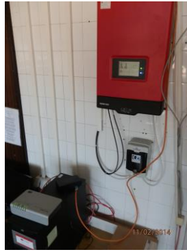
Fig. 3 Inverter and ancillary equipment for the monitoring and data acquisition of PV solar power plant at FSM in Niš
