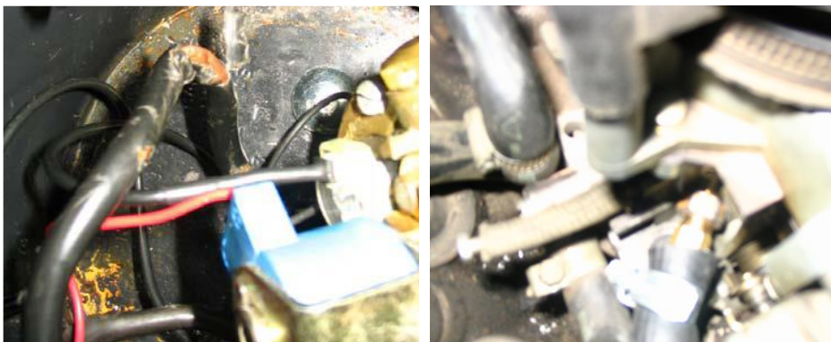
Fig. 6 Mechanically damaged pipe during installation Fig. 7 Larger hose diameter than the connection leading to LPG leakage
