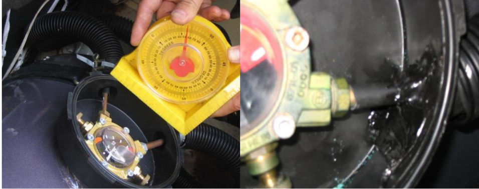
Fig. 2 The angle of the multivalve is not 30° Fig. 3 Ventilation passage closed
